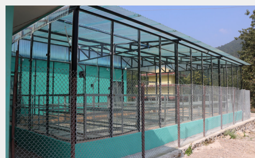
Newly built solar drying facility
